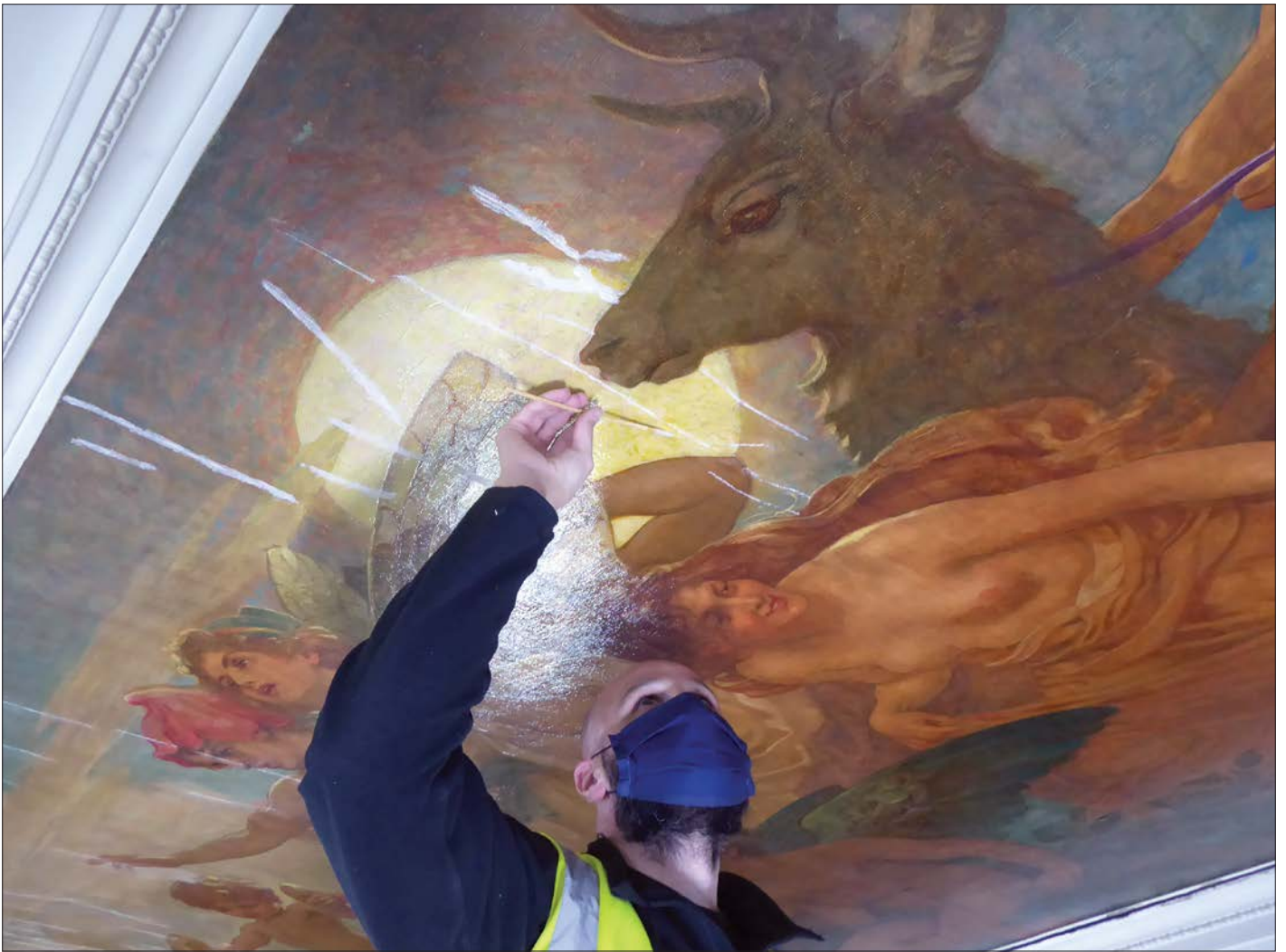
Drapers Hall, London 2021 showing careful filling to one of the marouflage ceiling panels prior to retouching and revarnish
