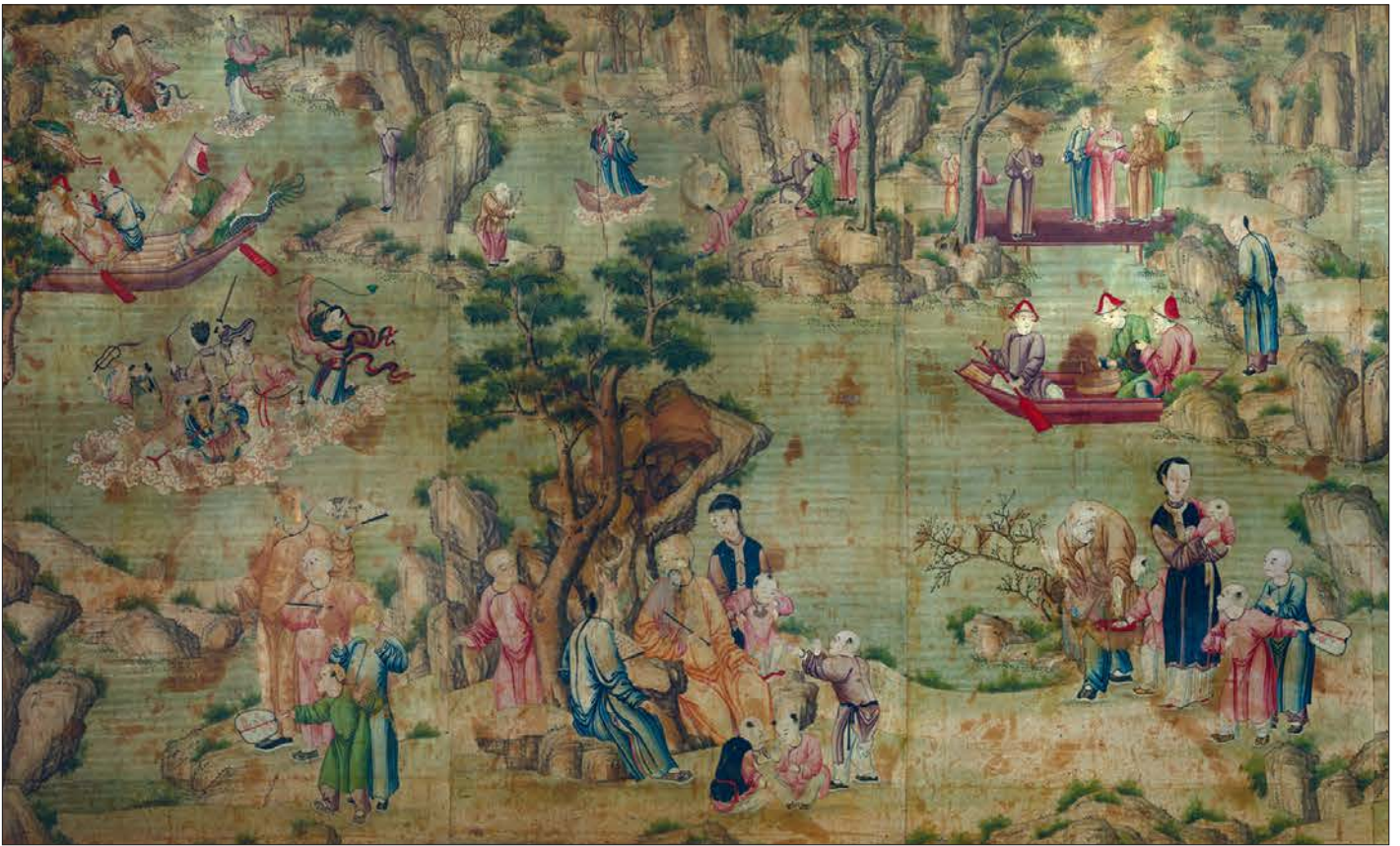
The long wall of the Adelaide Corridor, depicting the Dragon Boat Race, a scene of mythology. Note the brown stains, especially the square radiator-shaped stain (bottom right over page) where the wallpaper was varnished beneath
