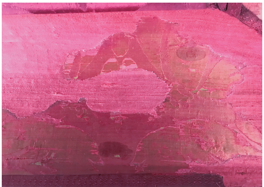
Fig. 17 Large area of infill patches on the foot cornice.
