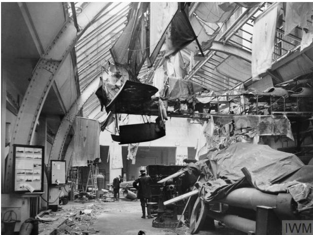
Air raid damage to the Naval Gallery at the Imperial War Museum, London, 31 January 1941. © IWM (MH 127)
