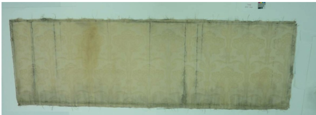
Figure 3 Black "dribbles" and overall discolouration.
